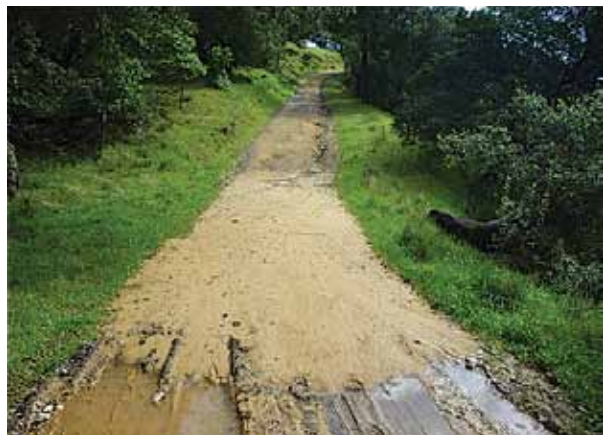
Figure 3.19 Sediment from erosion of the road bed is deposited in a natural dip. Frequently placed drainage dips could have minimized this erosion.
