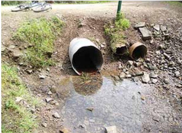
Figure 3.39 Stream crossing with culvert. Note the two smaller pipes, which were undersized and became plugged with sediment.
