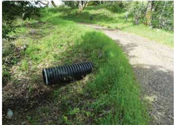
Figure 3.40 Recently installed plastic pipe. Outlet is "shotgunned," leading to erosion at the outfall.
