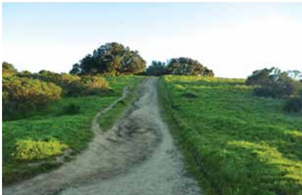
Figure 3.8 Erosion of fall line segment of a fire road. Notice that the lower portion of the road is in a through-cut.
