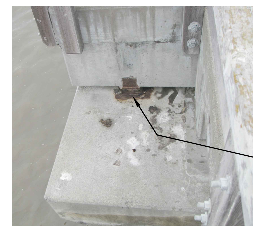
HARDWARE CORROSION AT EXPANSION JOINT HARDWARE REPAIR M1 S9
