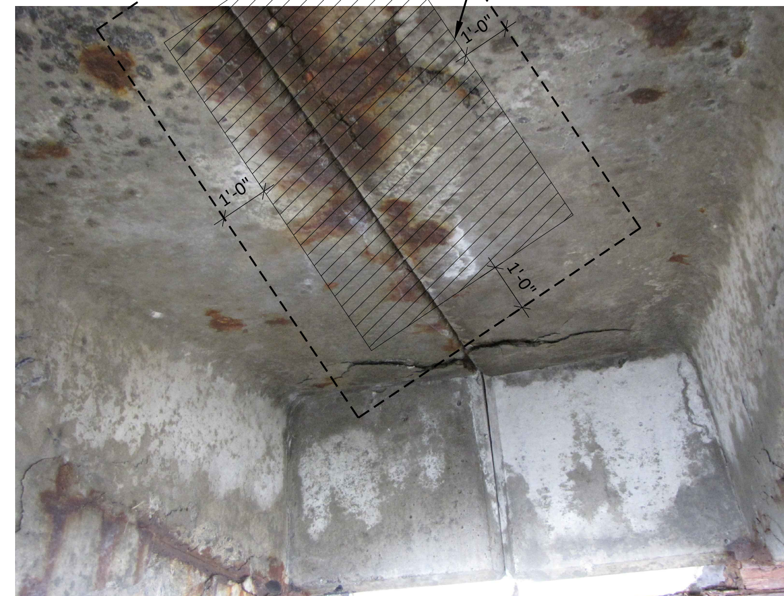
TEE CRACKING AT DECK JOINT DECK JOINT REPAIR D3 S9
