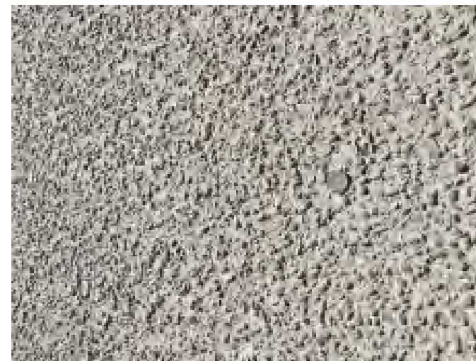
HIGH SEVERITY WEATHERING
