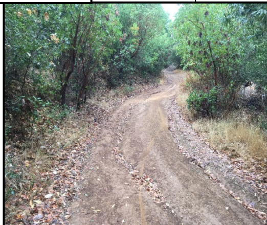
Photo 3: Rutting in Ponti Fire Road
